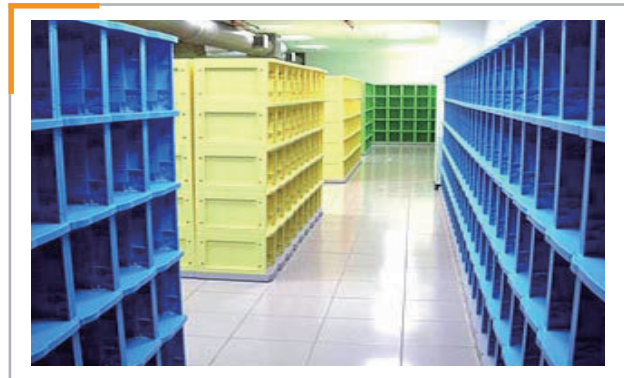
Taipei Power Plant
